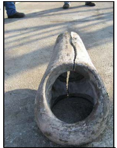
Failed Mooring Socket
