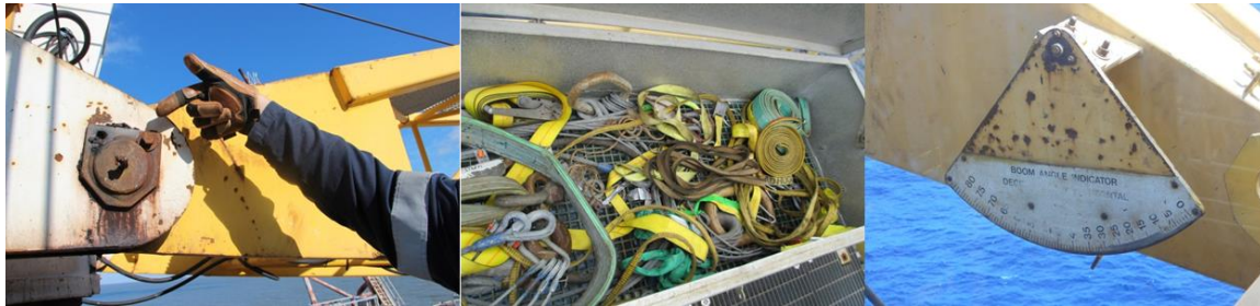
BSEE and USCG Inspectors identified missing bolt from the boom heel section on platform crane, poorly maintained lifting equipment, and numbers faded off of a boom angle indicator during crane risk inspections.
